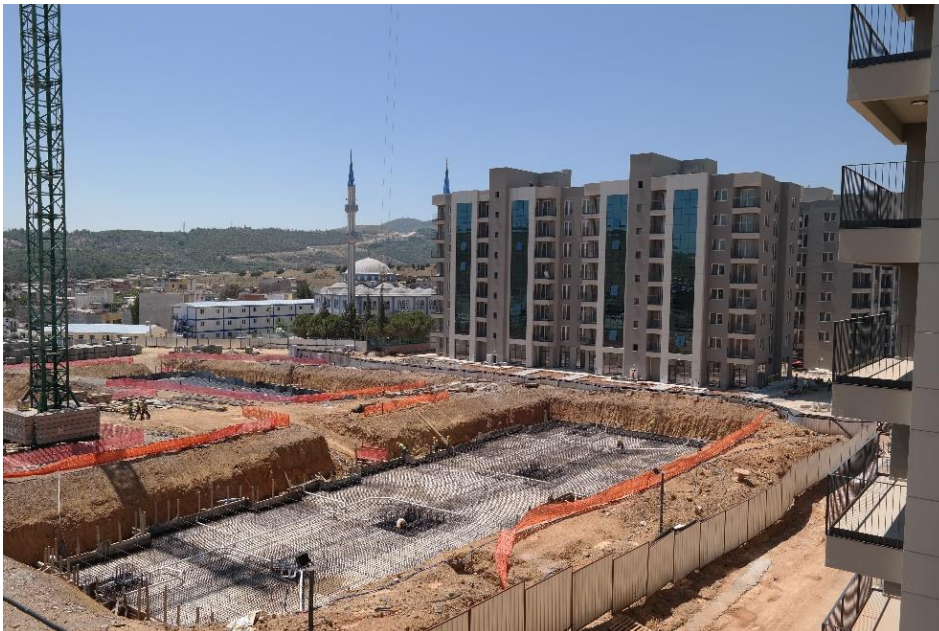
Figure 54. Constructions in the 1 st phase about to be completed and constructions starting in the 2 nd phase in July 2018
